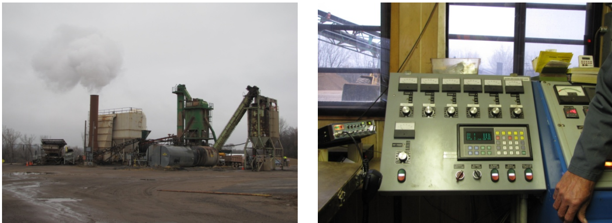
Figure 1: Crane Creek Batch Plant
